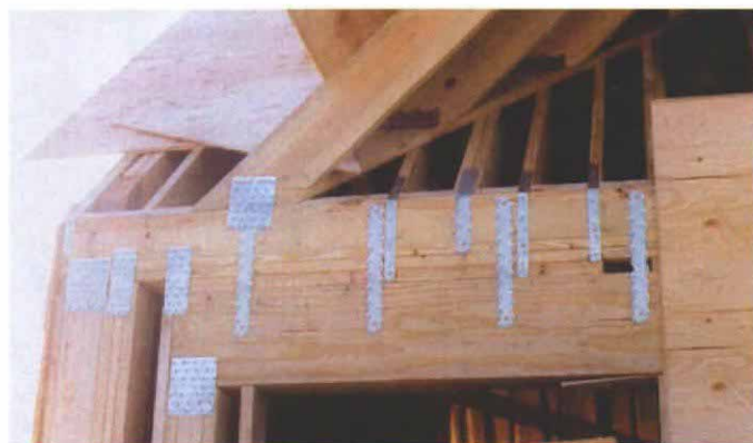
Hurricane straps. Typical of the detailing throughout the house, every rafter was fastened to the walls with galvanized metal straps.
