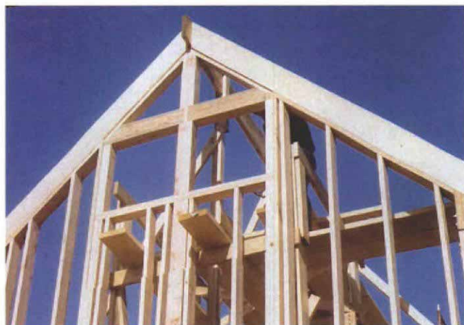
Shear wall. One of two shear walls in the house, this gable end was strengthened with 6x6 timbers that run from the foundation to the rafters. The wall was sheathed on both sides with \frac{3}{4} -in. plywood.
