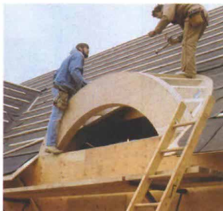
Plywood header. The header for the arch top kitchen window is made of seven layers of \frac{3}{4} -in. plywood cut to fit the window's curves.
